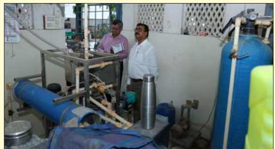
At the Water Plant (RO)
